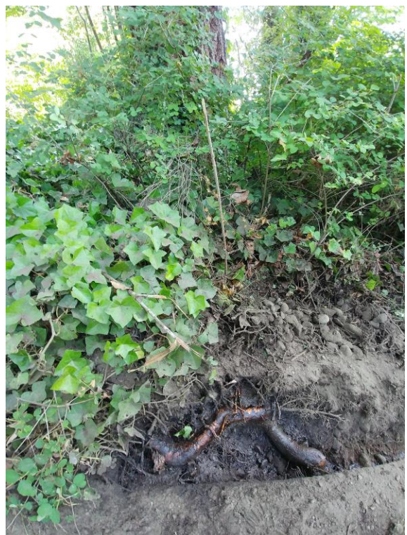
Photo 3 The Douglas fir tree behind the root found from the maple. This root is below the grade of the pavement and three feet long.
